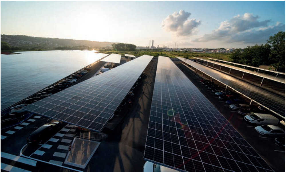
• Photovoltaic power plant at the Safran Nacelles industrial site, Gonfreville-L'Orcher, France.
